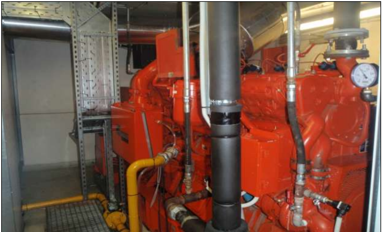
ATHENS HILTON SITE: VGF H24GLD GE-WAUKESHA GAS ENGINE
